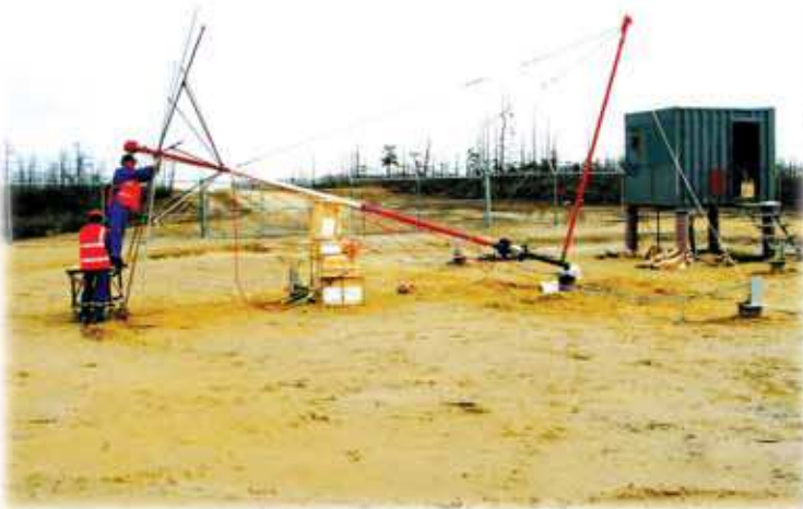
▲ Installation of AZM-8 antenna by Technomarine's specialists on General Dynamics site, Project Sakhalin-1
