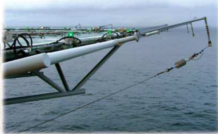
▲ Antenna «Koltso-2» and Homing NDB «Privod-3» on oil-and-gas drilling plate of Exxon Neftegas Limited (USA), Sakhalin shelf
