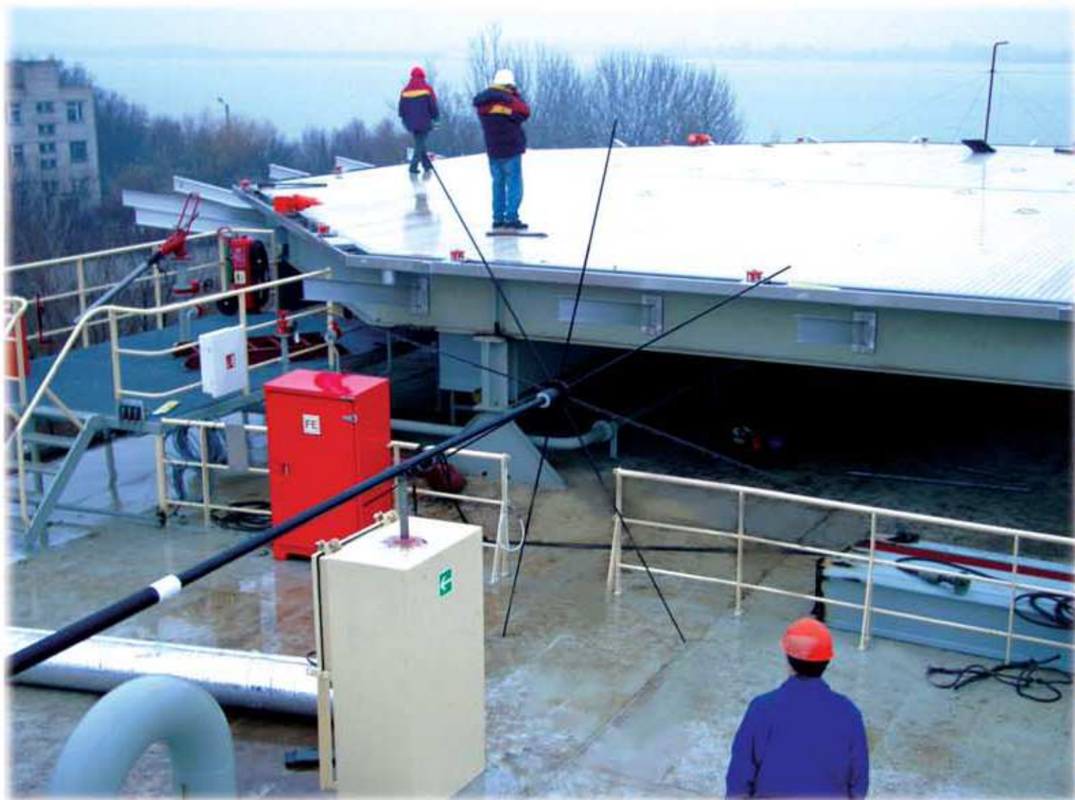
▲ Helicopter homing equipment «Privod-3» on CASTORO-12 pipelayer ship of Saipem SpA company (Italy)
